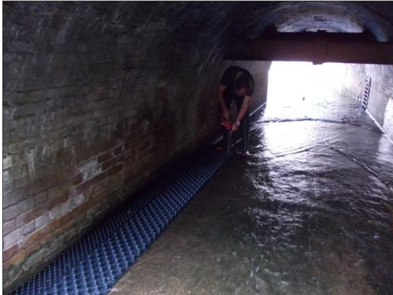
Figure 11: Attaching a row of eel tiles to the riverbed at Clattern Bridge
