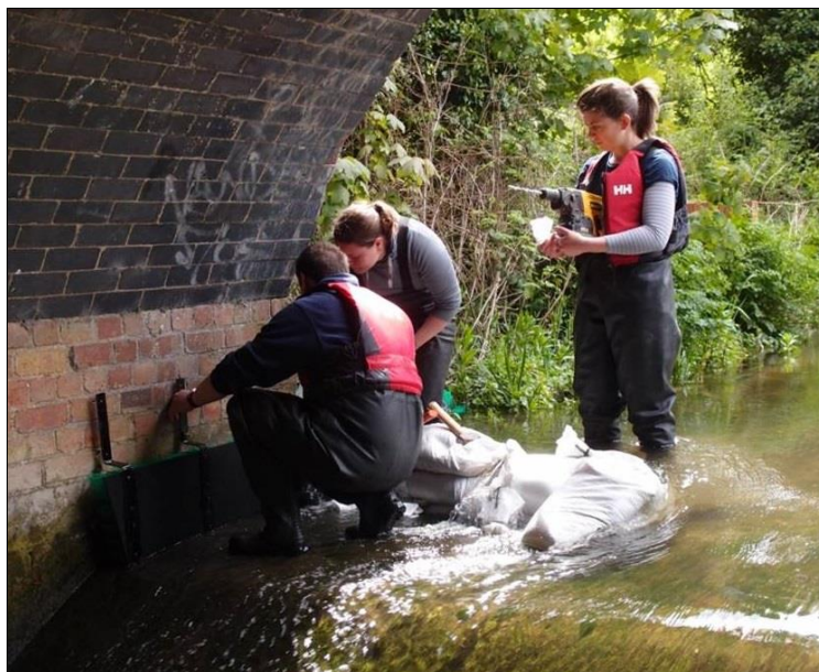
Figure16: A 'bristle board' eel pass being installed on the River Darent with the North West Kent Countryside Partnership.
