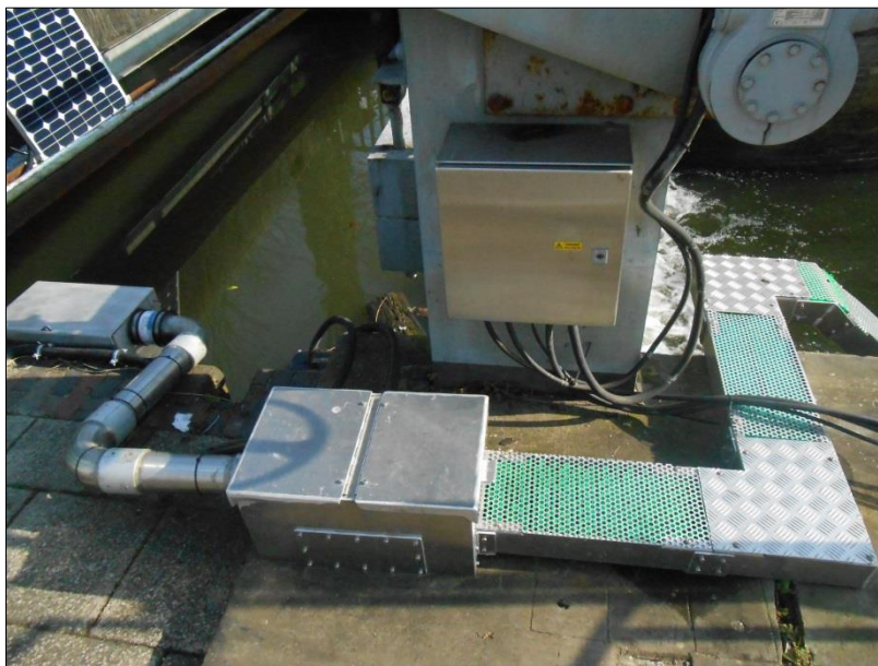
Figure 8: The eel pass installed by Aquatic Control Engineering at Stoney Sluice.
